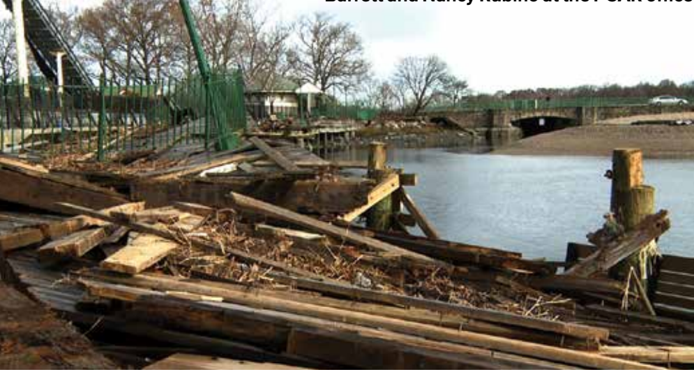
The devastation caused by Hurricane Sandy in 2012 at Rye Playland.
