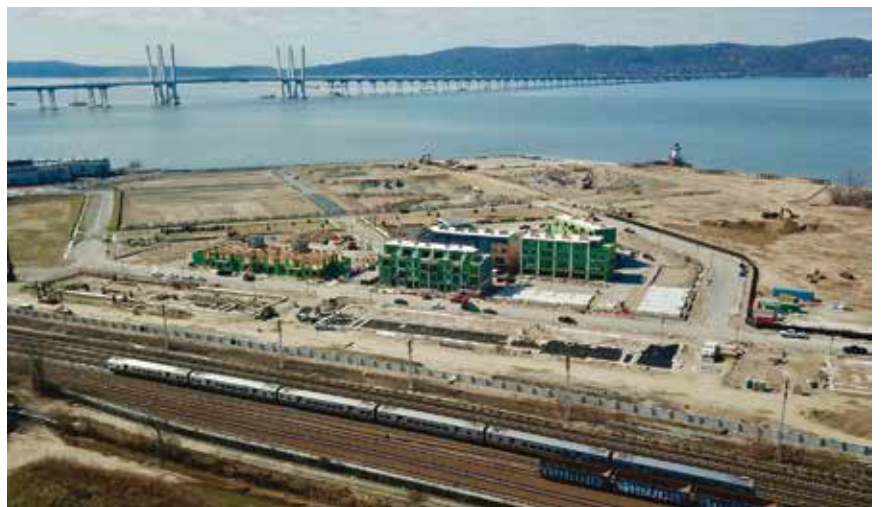
An aerial of the construction taking place at the Edge on Hudson project.
