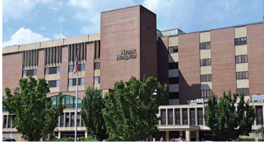
Nyack Hospital is set to commence its ambitious Care Transformation Project that includes the construction of a two-story addition, which will double the size of the existing Emergency Department and add a new Medical Village. The hospital secured CFA funding for its Transitional Care Unit on the fourth floor 4-Maze Nursing Unit.
