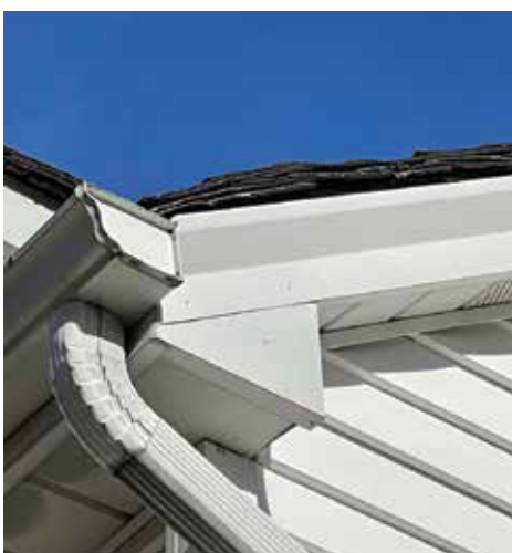
Multiple layers of roof shingles, which can weigh down heavily on roof rafters. (Photo courtesy of Pillar to Post Inspections)
