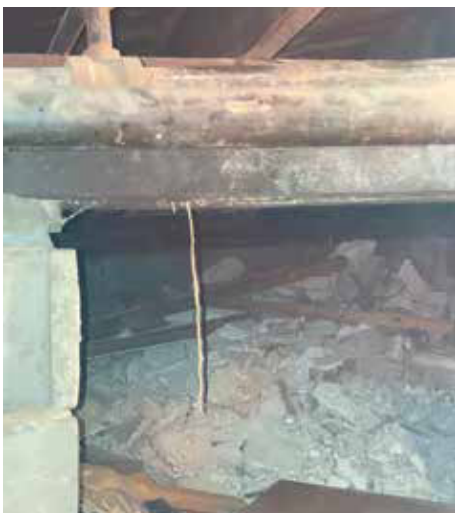
Missing stones and mortar deterioration on the side of a home (Photo courtesy of Pillar to Post Inspections)
