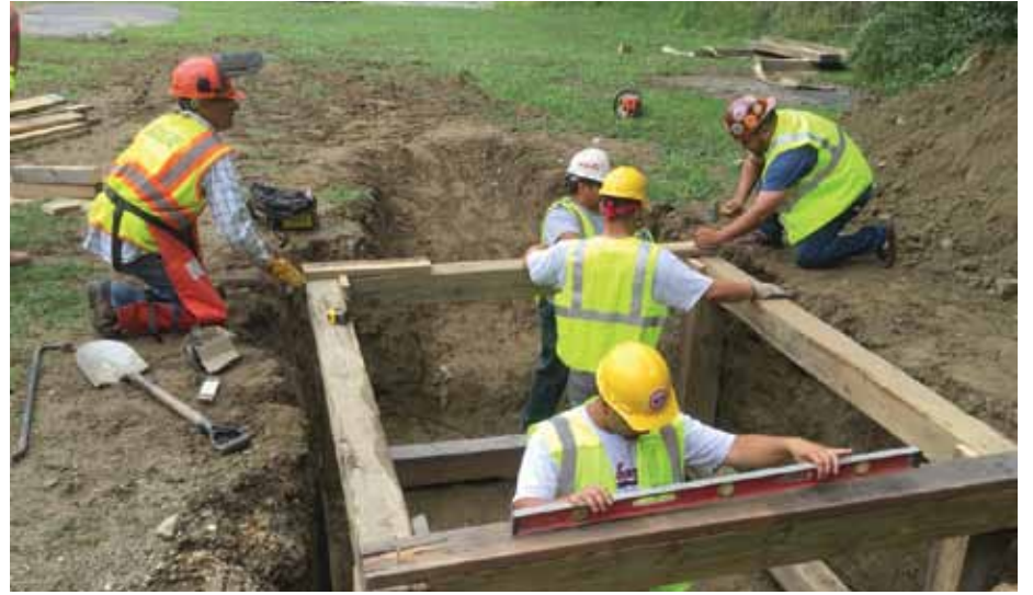
Local 60's Trench & Excavation Safety class is conducted outside the training center facility.
