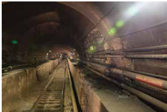
The North River Tunnel under the Hudson River connects New York and New Jersey and carries Amtrak & NJ TRANSIT passengers making 200,000 daily trips.
