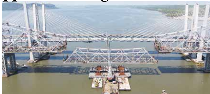
The 532-foot section of the center span was lowered onto a barge.
